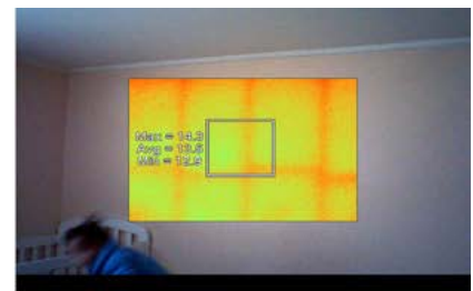
c Main bedroom south-west: no insulation
