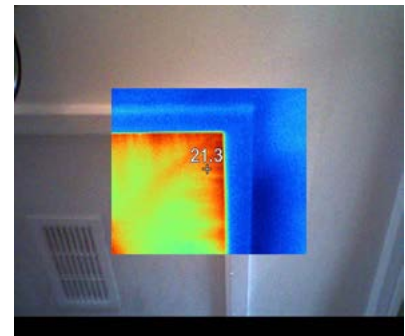
Leakage around roof access hole
