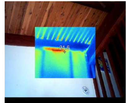
Leakage between architrave and gyprock
