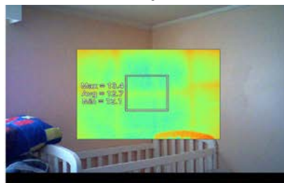
b Main bedroom south: no insulation
