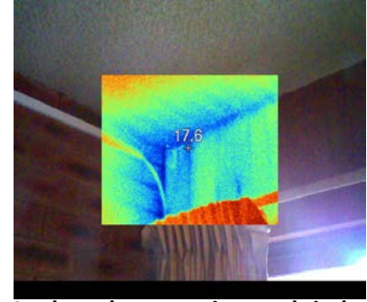
Leakage between internal timber cladding, brickwork and ceiling
