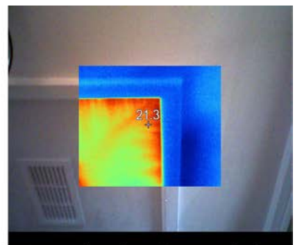
c Uninsulated roof access hole (and air leak)
