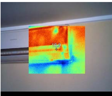
Leakage around air-conditioner
