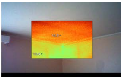
a Main bedroom south: thin ceiling insulation, no wall insulation
