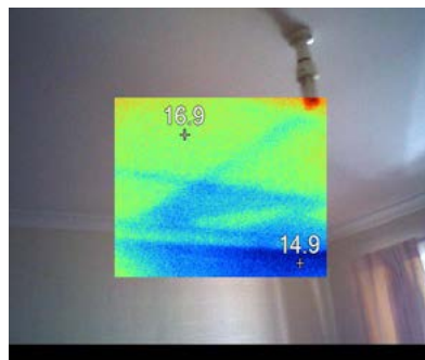
Patchy ceiling insulation 5 October 2012, 10:36:38am
